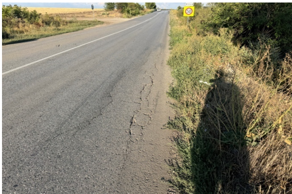
Figure 72 – Clearly visible longitudinal crack.
