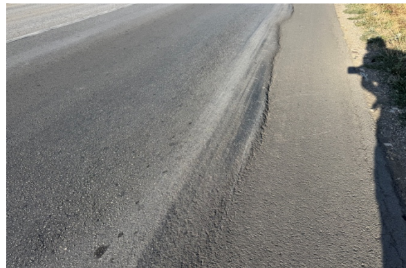
Figure 73 – Poor-quality asphalt at one of the patches.
