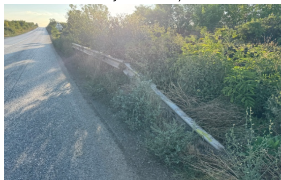
Figure 30 – Example of vegetation clearing behind the road maintenance base – left traffic lane in the direction of travel (town Knezha ← town Byala Slatina).
