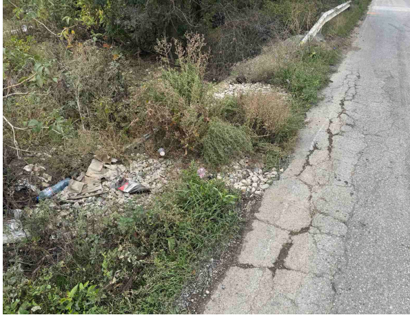
Figure 22 – Condition of the surface above the culvert.
