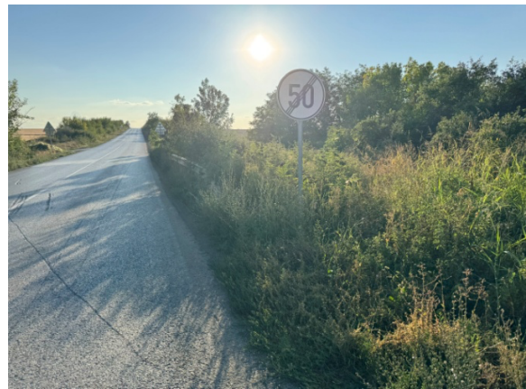
Figure 37 – Condition of the shoulder – right traffic lane in the direction of travel (town Knezha → town Byala Slatina).
