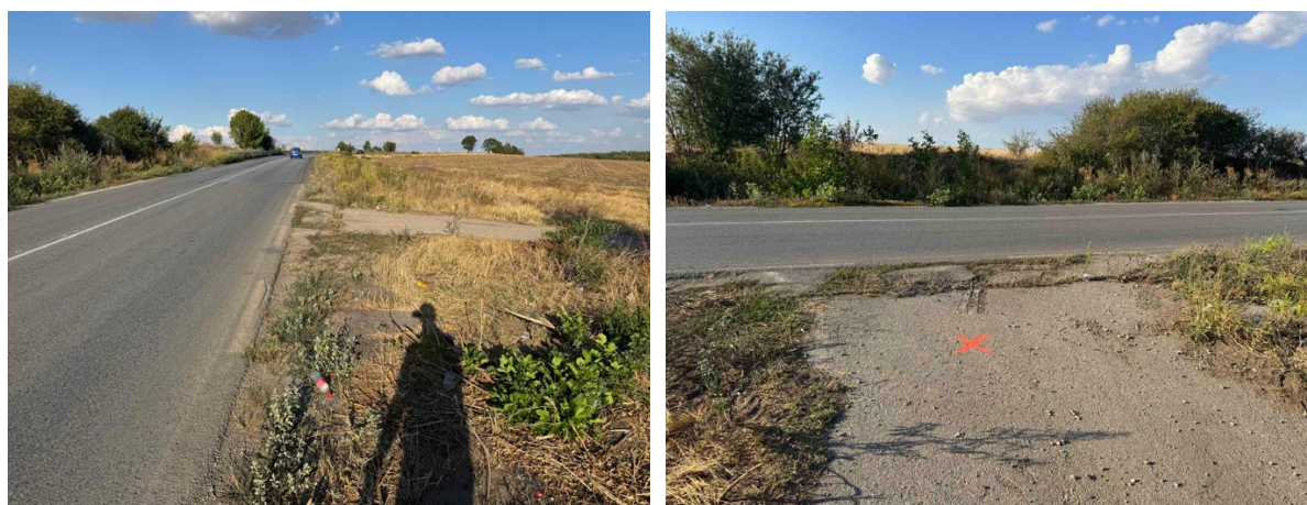
Figure 14 – Direct joining of an unregulated dirt road to the alignment of republican road II-13. In the PPBD (old project), the installation of road sign B2 was planned for this road (at km 65+831), while the dirt road is located at km 65+824.
