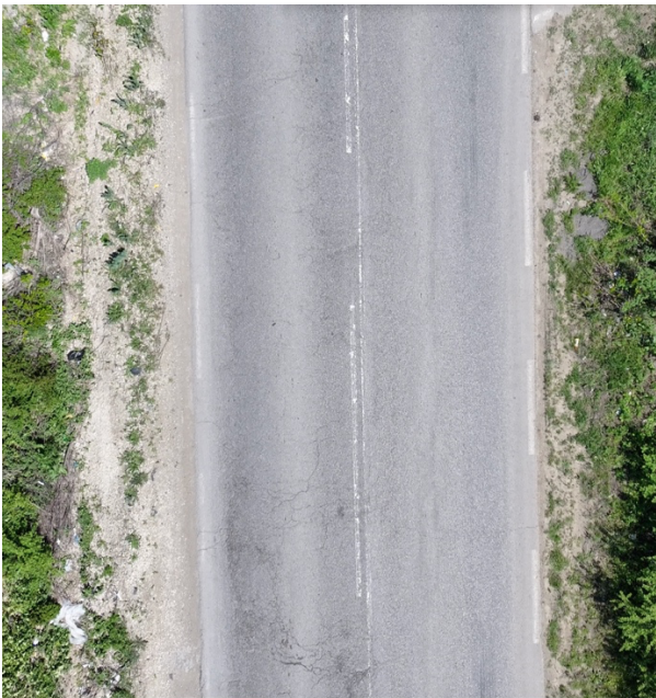
Figure 51 – Condition of the road marking as of May 2025 before the safety measures for the UKPTP were implemented – footage captured by the remote sensing method.
