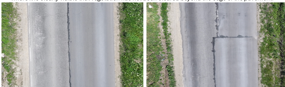
Figure 32 – Condition of the edge of the pavement, footage captured by the remote sensing method. The survey was performed by the EUCTP team in April 2025.
