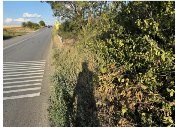
Figure 35 – Condition of the shoulder – right traffic lane in the direction of travel (town Byala Slatina → town Knezha).
