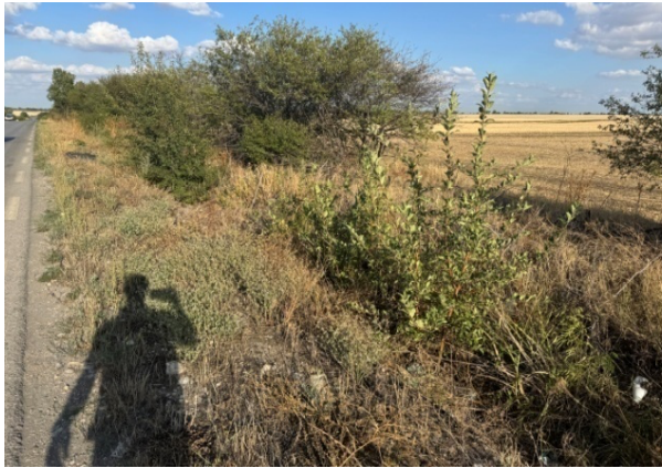
Figure 34 – Condition of the shoulder – right traffic lane in the direction of travel (town Byala Slatina → town Knezha).
