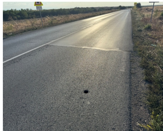
Figure 48 – Condition of the edge line marking the end of the carriageway (right lane, direction from town Knezha to town Byala Slatina). The photo was taken in September 2025 after the safety measures for the UKTP were implemented.
