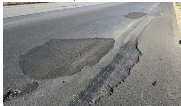
Figure 75 – Zone with clearly visible lateral shoving and a formed step with a height exceeding 7 cm.
