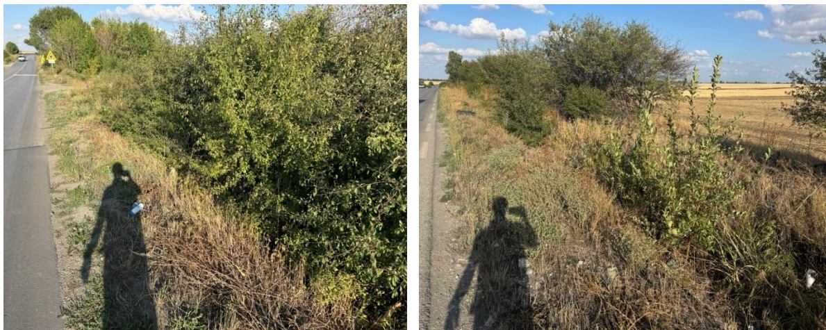
Figure 38 – Condition of the slopes in the studied section (direction from town Byala Slatina to town Knezha).
