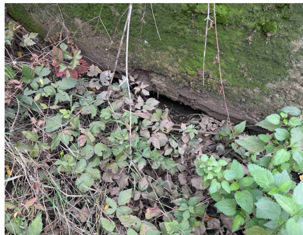
Figure 25 – Condition of the culvert – view from the north side of the road (direction of travel from town Knezha to town Byala Slatina).
