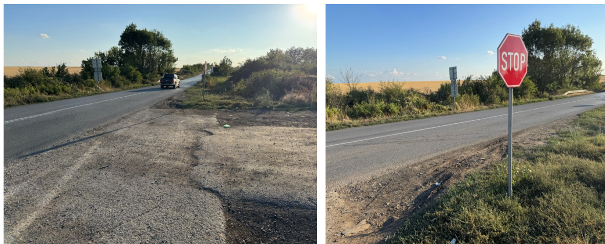
Figure 18 – The presence of asphalt pavement at the turn-off for the agricultural/forest road and the presence of road sign B2 on the left side in the direction from town Byala Slatina to town Knezha were established. Sign A26 is missing.
