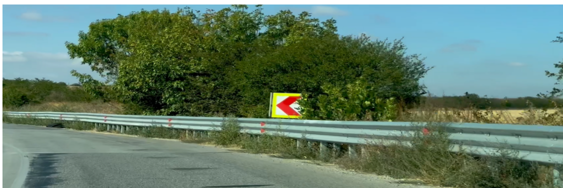
Figure 31 – Road restraint system in the curve in the direction from town Knezha to town Byala Slatina, where it is clearly visible that vegetation has not been cleared beyond the edge of the pavement.
