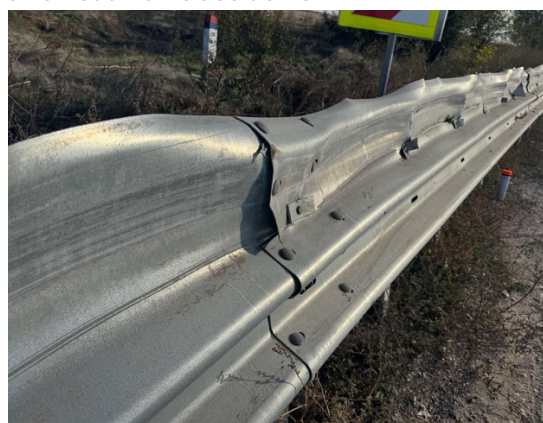
Figure 66 – Condition of the road restraint system after the safety measures for the UKPTP were implemented. From the traces of numerous impacts, it is clearly evident that the cause of the road accidents is complex and the restraint system is not the best solution.
