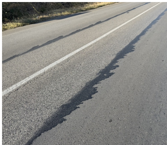
Figure 77 – Difference in the aggregate grading between the old and the new asphalt. The old grading is Type B, while the new grading is Type A.
