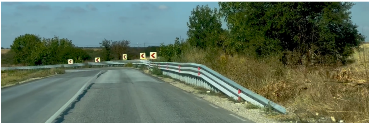
Figure 61 – Initial element of road restraint system at km 66+010 (direction of travel from town Knezha to town Byala Slatina) before the safety fence, which does not comply with the requirements of point 2.2 “Execution of initial and final elements of road restraint systems” to Ordinance No. RD-02-20-1-RRS. It must be replaced with a single terminal.
