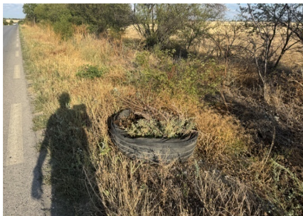
Figure 27 – Condition of the shoulder – right traffic lane in the direction of travel (town Byala Slatina → town Knezha).
