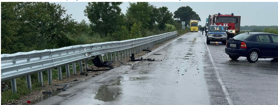
Figure 64 – Photo reflecting the current condition of the road restraint system on 25.05.2025 in the zone of the section with concentration of road traffic accidents.
