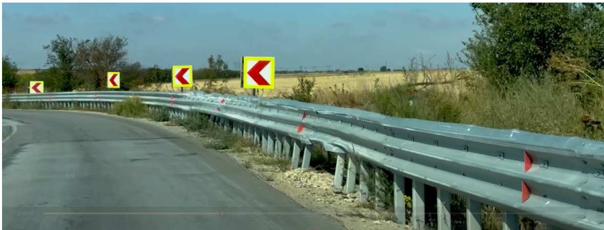
Figure 62 – Damaged road restraint system as a result of a road traffic accident, located on the right side of the left curve in the direction of travel from town Knezha to town Byala Slatina.
