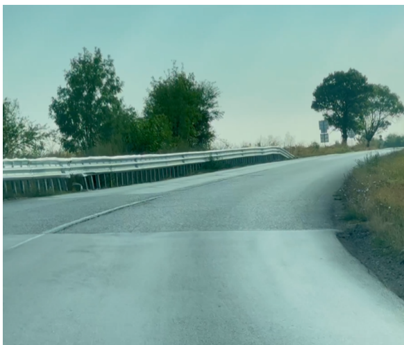
Figure 76 – Condition of the asphalt pavement in the curve.
