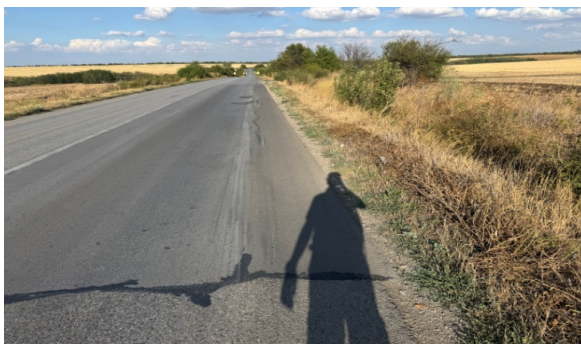
Figure 74 – General view before one of the patches, at which lateral shoving is observed.
