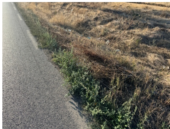
Figure 28 – Condition of the shoulder – left traffic lane in the direction of travel (town Knezha ← town Byala Slatina).
