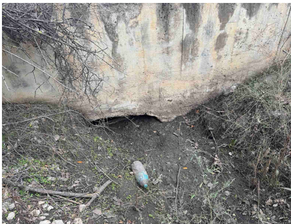
Figure 24 – Condition of the culvert – view from the south side of the road (direction of travel from town Byala Slatina to town Knezha).
