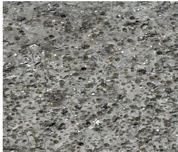
Figure 56 – Condition of the road marking as of 10 August 2025.
